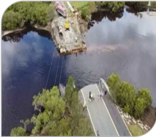
The loss of this causeway caused significant impacts for the White Patch community in 2022.
